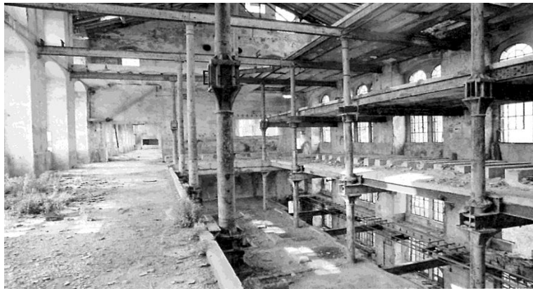
Figure 8. Ferrara, Sugar refinery of Pontelagoscuro,. Internal view with particular cast iron pillar and archway slab .
