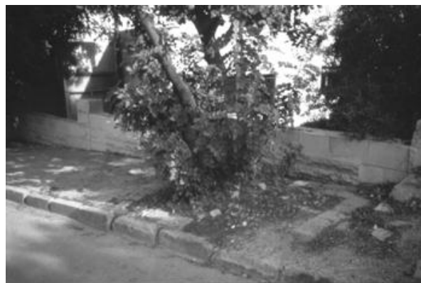
Figure 2. A scene often seen on Ammani's streets, a sidewalk interrupted by a large tree. Source: CSBE, 2004.
