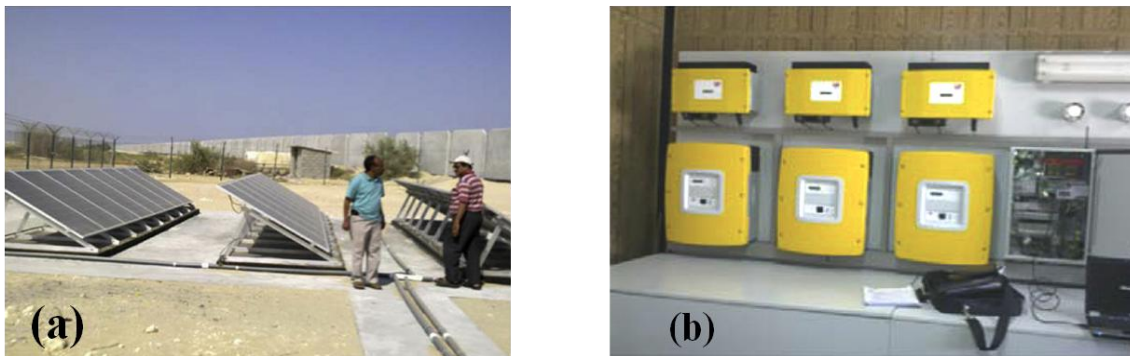
Figure10: View of: (a) the PV arrays installed at KFUPM beach, (b) PV control system installed inside the control room (Rehman & El-Amin, 2012).
