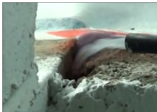
Figure 11: Pre Completion Air Tightness penetration, Block Sill to Column (O'Riain 2012)
