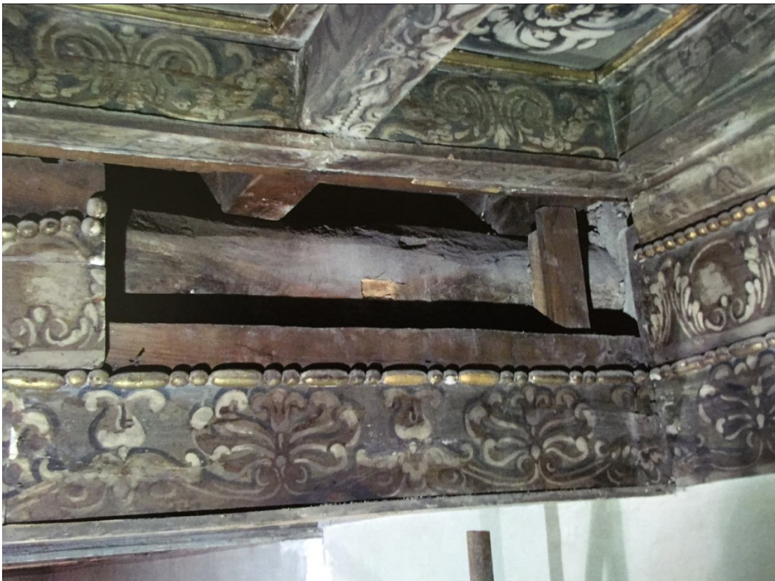
Fig. 3: Detail of the Ceiling. The Structure Made by Wooden Beams was Enclosed in a Series of Decorated Planks
