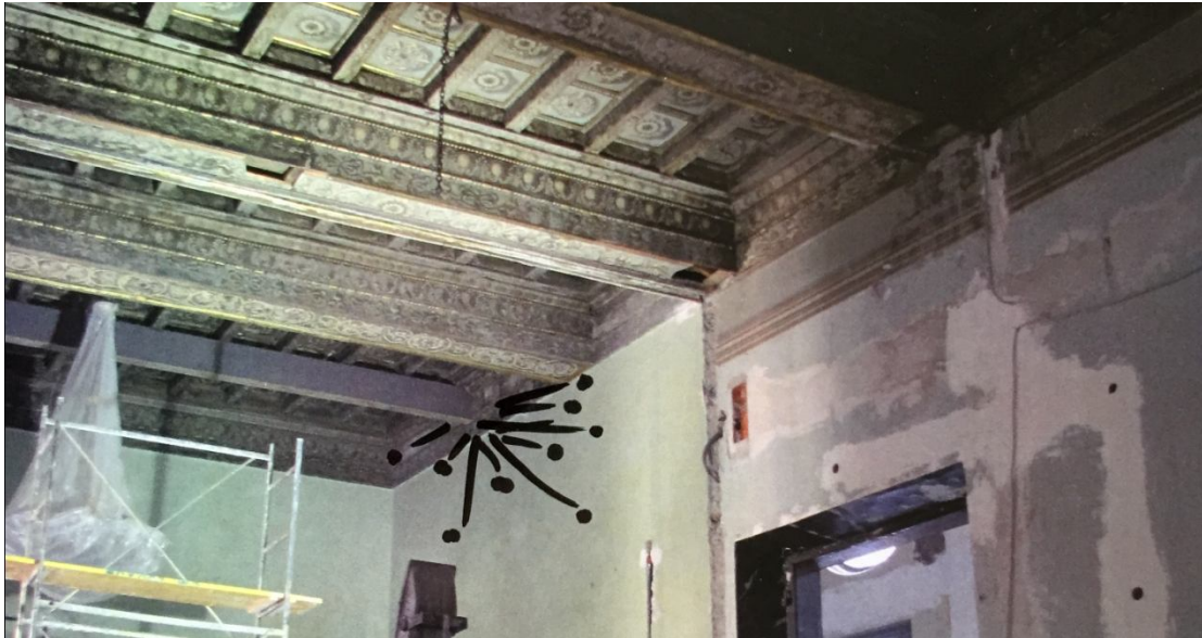
Fig. 1: Wooden ceiling. Clearly Visible, on the Left There is a Steel Beam.
