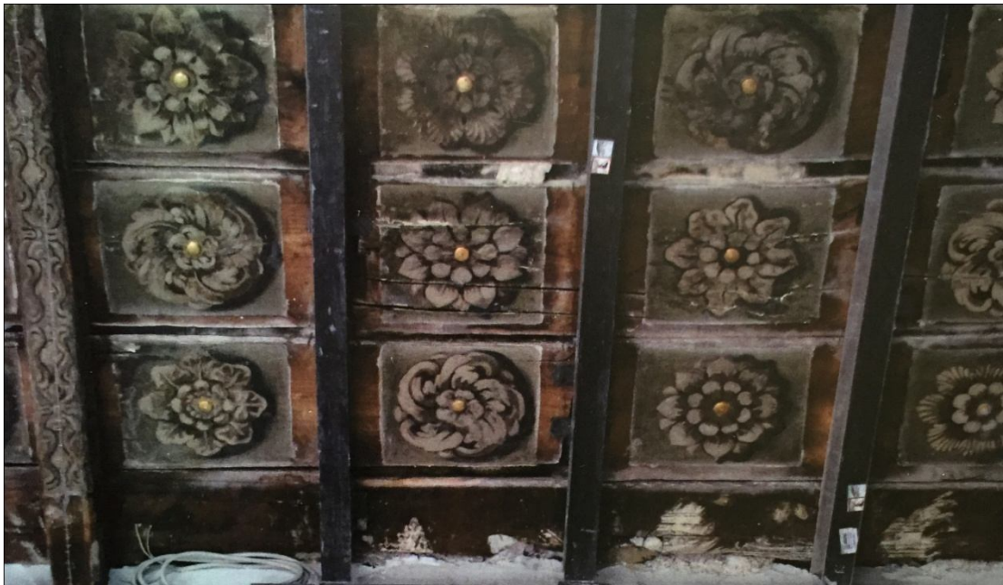
Fig. 5-6: Top. The Irremediably Damaged Secondary Wooden Beams are Replaced with Steel Ones, the Next Step (Bottom) Is to Use the Same Technique Used in Ancient Times for the Primary Beams that Were Covered by Applying Decorated Planks
