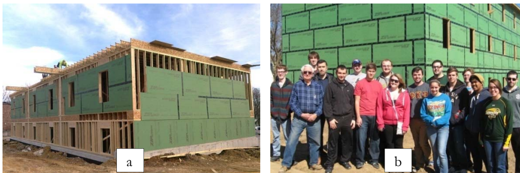
Figure 3: Visiting of Timber Frame Construction site in Rolla, Missouri by ArchE 2103 Students in Spring 2014 term (Yildirim, 2014a)
