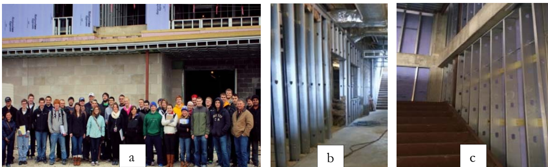
Figure 4: Visiting of Missouri S&T Biochemical Building (Bertelsmeyer Hall) construction site in Rolla, Missouri by ArchE 2103 students in spring 2014 term
