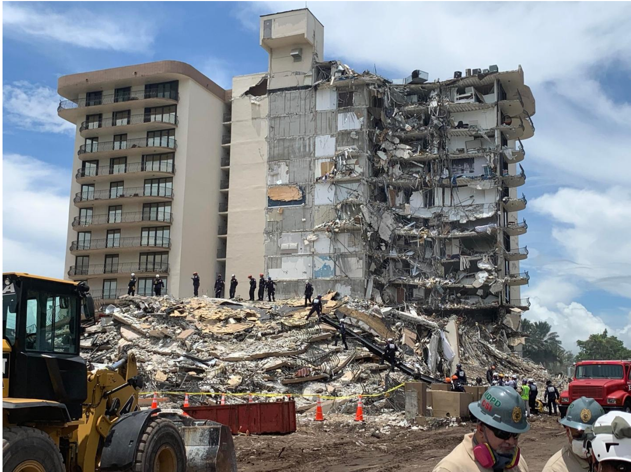
Figure 2. Search and rescue teams at the site of the collapse. Photo: National Institute of Standards and Technology (NIST, 2021).
